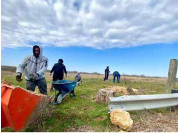
Building a new pocket wetland on the Fort Worth Prairie. We removed invasives around the new wetland site, which is near the entrance and was impacted, and reseeded it with carefully-sourced native grasses and forbs.
